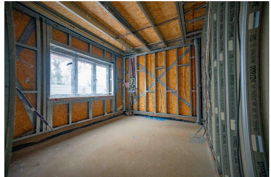
UNihouse on-site as installed, internal image
